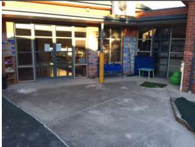
Rear of the existing building, footing exposure as requested could not be conducted here without concrete cutting.
